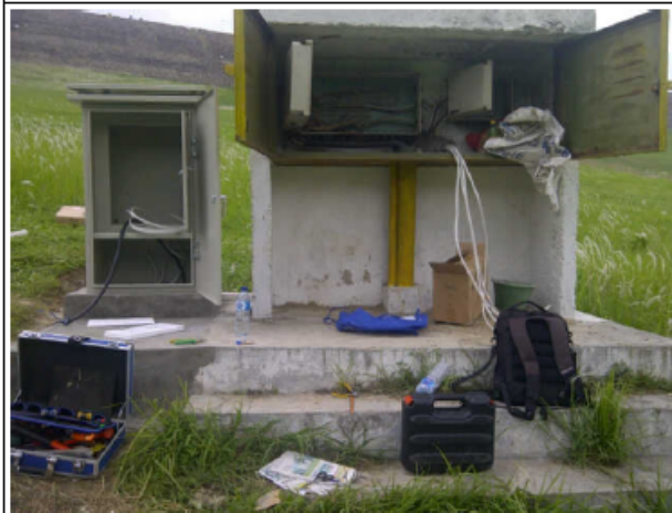
Outdoor Enclosure, Jatiluhur Dam, Telemetri Dam Safety, Balai Bendungan, DOISP Loan IBRD 2014
