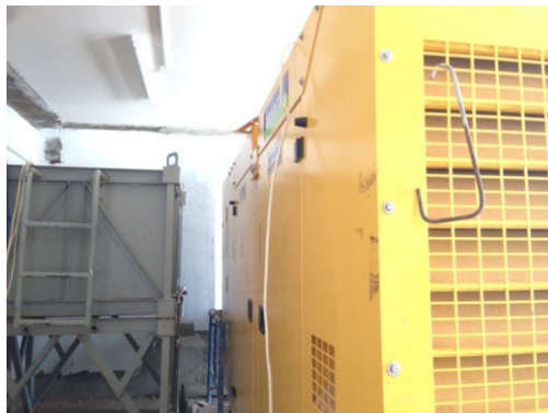
Generator Listrik & Fuel Tank
