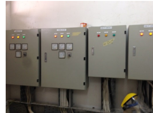
Panel Listrik Lantai 2
